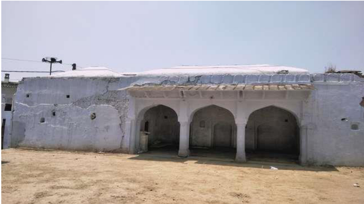
(Fig 2 Remains of the old buildings of graveyard compound in Manikpur (Physical Survey)
